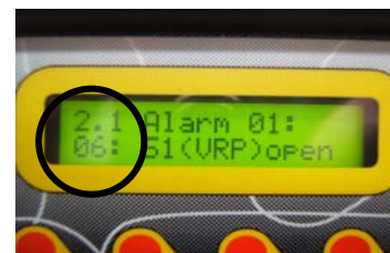
Last alarm was Fault code 06
